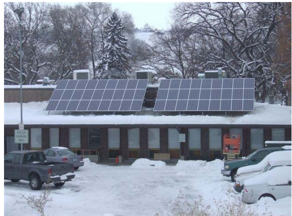
Solar array on the Pendleton State Office Building
