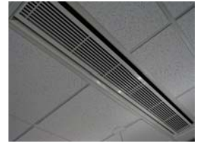
The chilled beams in the first floor lobby of the ESOB. They look like traditional vents in the ceiling.
