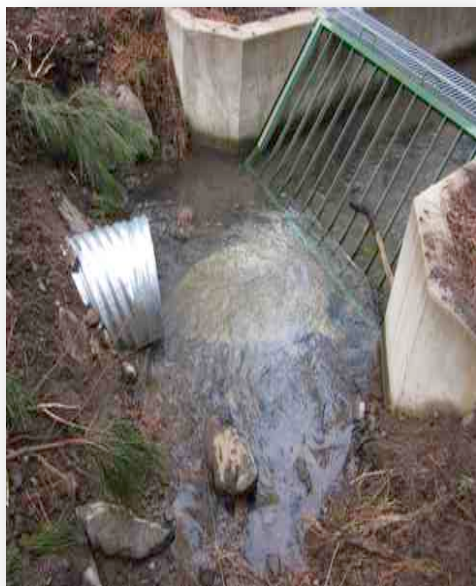
Fish passage project showing the installed culvert and smooth flow area for fish to be diverted through the escape route at the fish screen.
