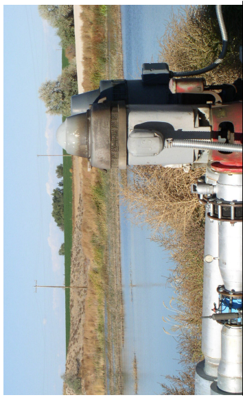
Pumping irrigation water out of a wetland constructed to clean tailwater.
