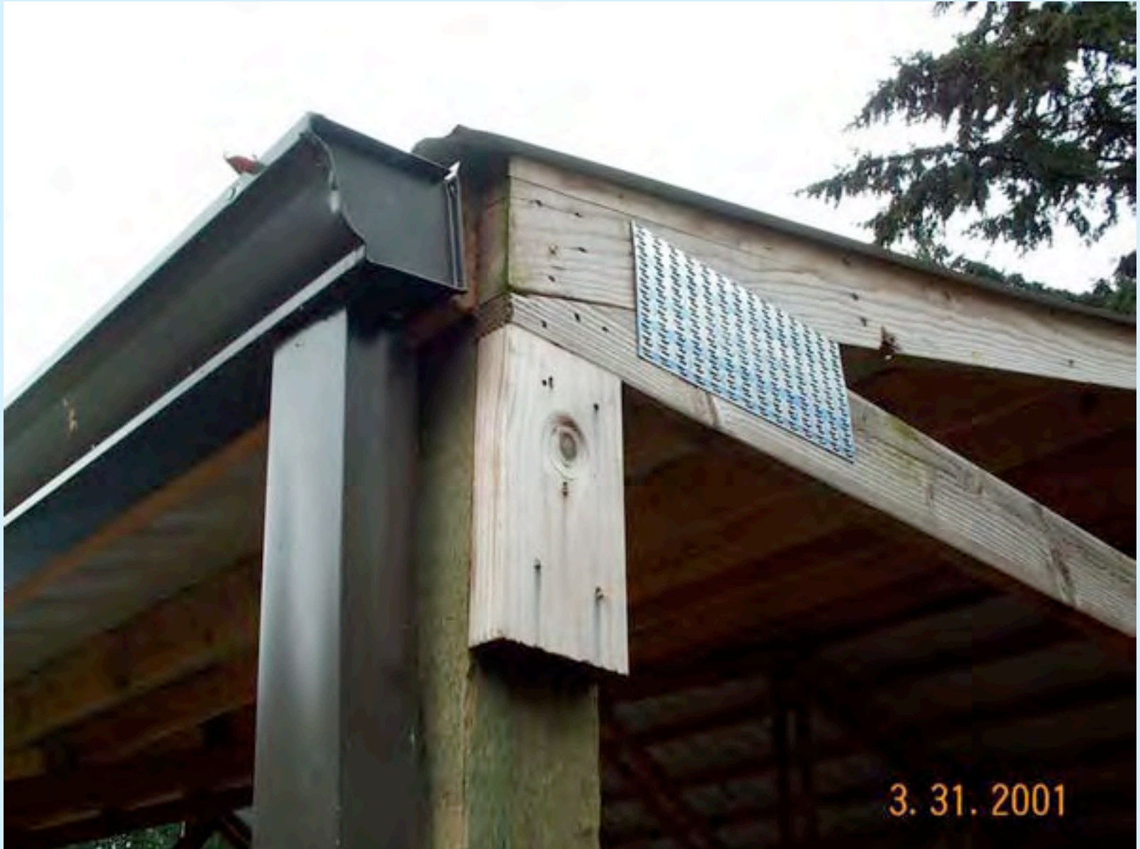
Industrial Size Gutters
