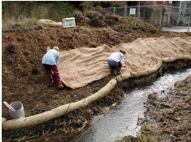
Erosion control matting and straw wattles are being installed in a riparian zone prior to planting.
