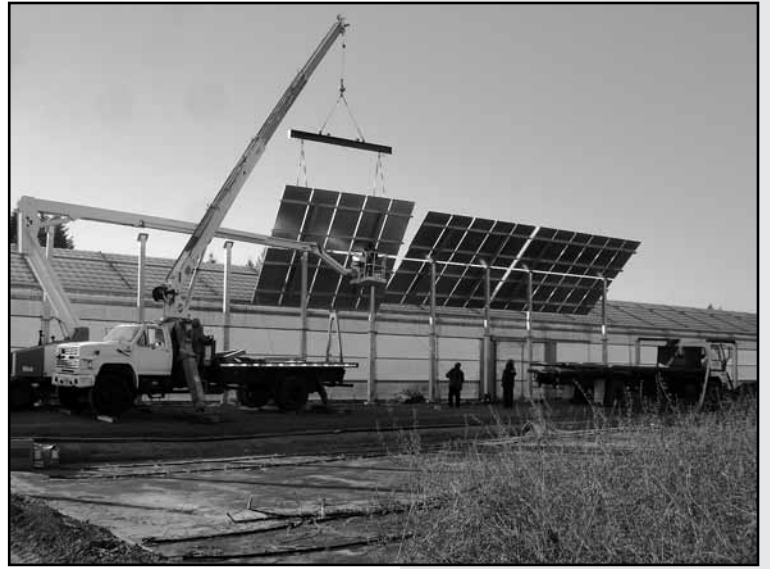
Above: A truck hoists solar collectors onto racks at Blooming Nursery in December.
